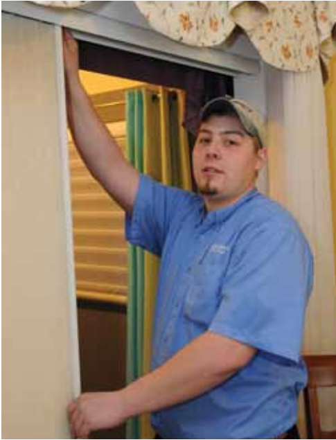
Robbie Babineau, part of Gordon's customercentric install team, fine tunes a insulating slider.
